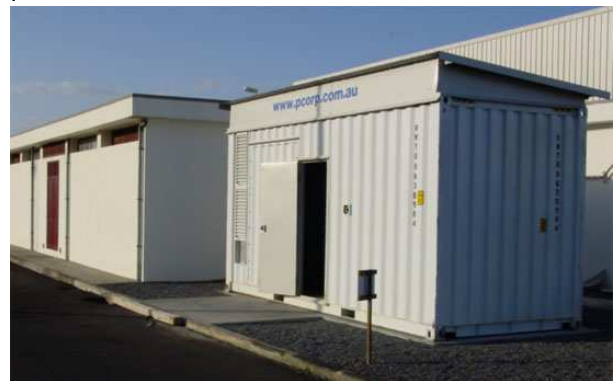
Figure 3 - PowerStore 500kW Container Outside view
