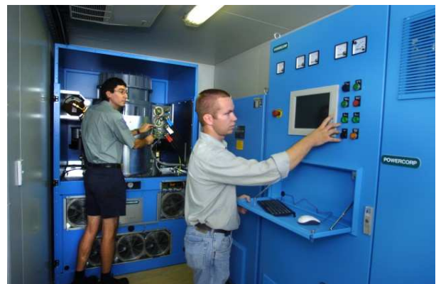
Figure 4 - Control Cabinet with SCADA Screen, inside of container
