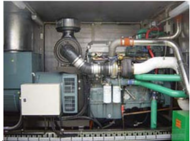
Figure 3 – Inside Low Load Diesel unit
