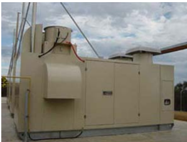
Figure 2 - Flywheel Installed within the containerised building
