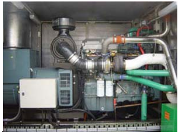
Figure 3 – Inside Low Load Diesel unit
