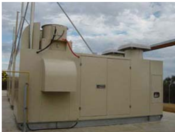
Figure 2 - Flywheel Installed within the containerised building
